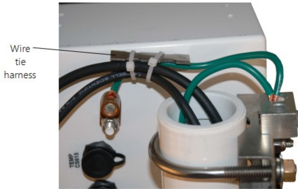
FIGURE 6-44. Cabling strapped to wire tie harness
