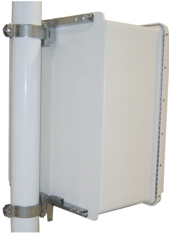
FIGURE B-7. Enclosure mounted on T107 pole
